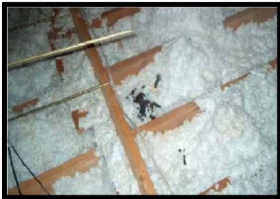
Feces & Disturbed Insulation
